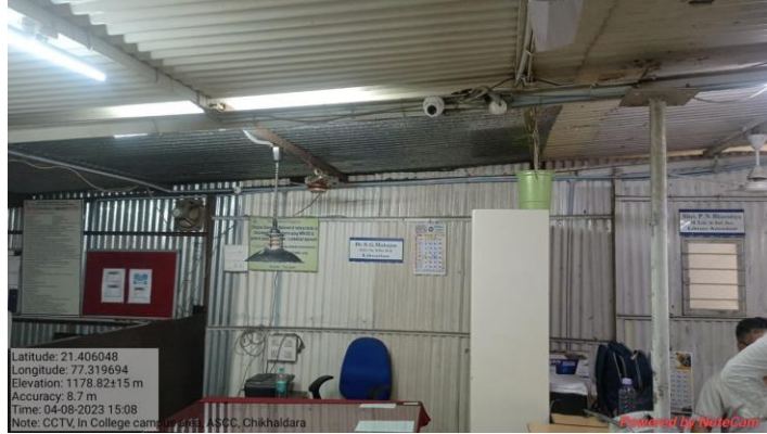
CCTV facilities, Library point 2, ASCC, Chikhaldara
