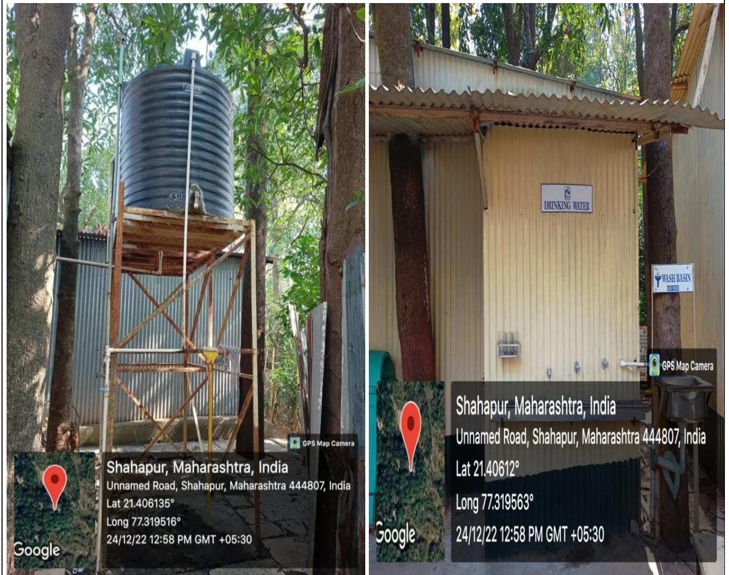
Water Tank for Drinking water at College Campus.
