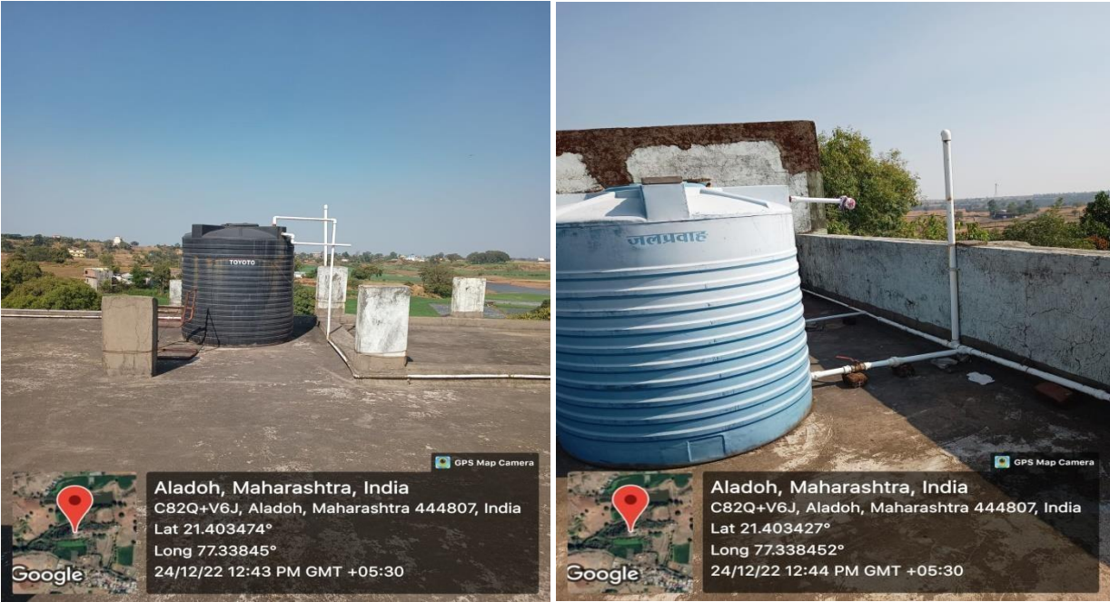
Water Tank for water supply at Women's Hostel at Aladoh Campus
