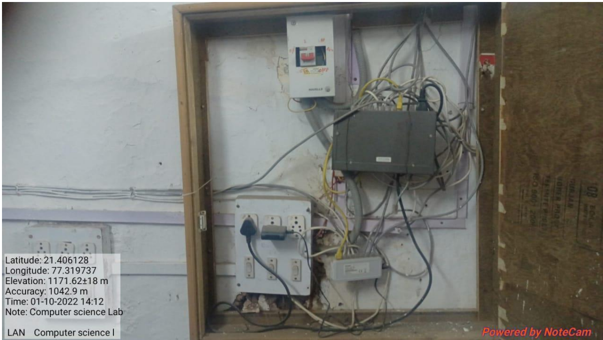
LAN facility at Computer Science laboratory
