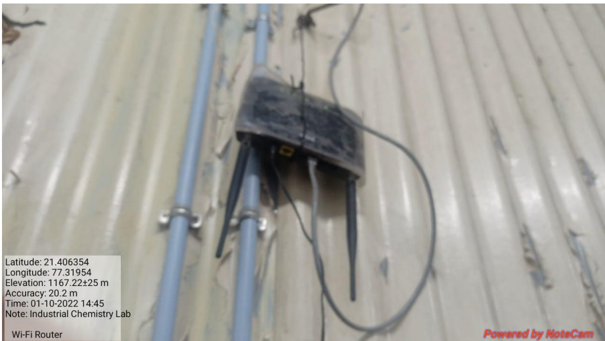
Wi-Fi Router at Department of Industrial Chemistry
