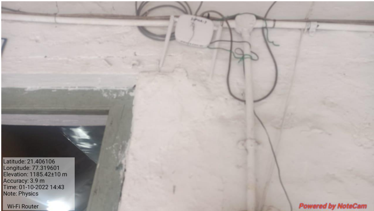
Wi-Fi Router at Department of Physics
